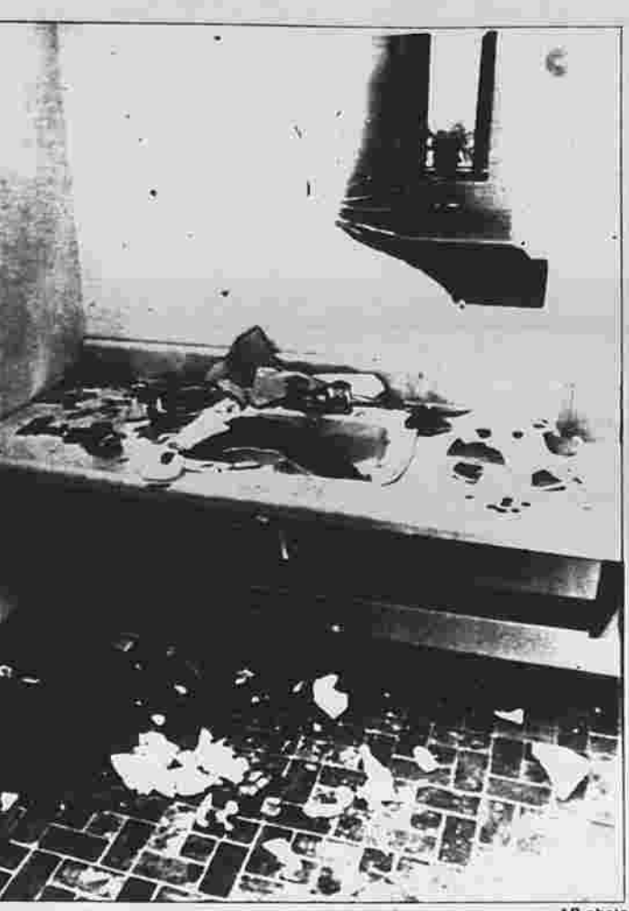
Signs of vandalism remain at East Lyme's Christ Lutheran Church Thursday afternoon. Vandals also ransacked through the East Lyme Junior High School, and damage is estimated at more than $75,000.
